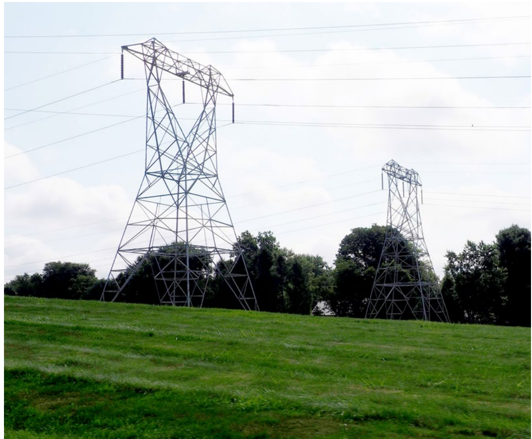
Greater coordination with utility providers such as PECO will help ensure Township residents and businesses have uninterrupted access to their services.
